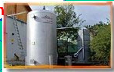
Biogas from Solidfermatation Process
